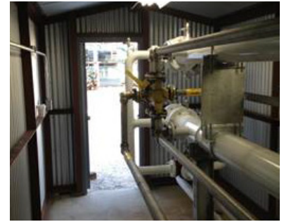
Dense plant topography of metal and concrete, tanks, walls, piping, structure, and buildings was not a problem for the wireless network.
