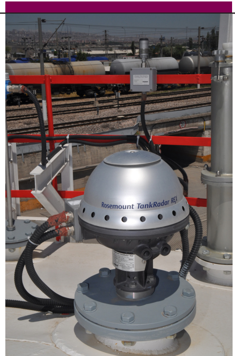
TankRadar Rex radar level gauge installed with the Smart Wireless THUM Adapter antenna unit.
