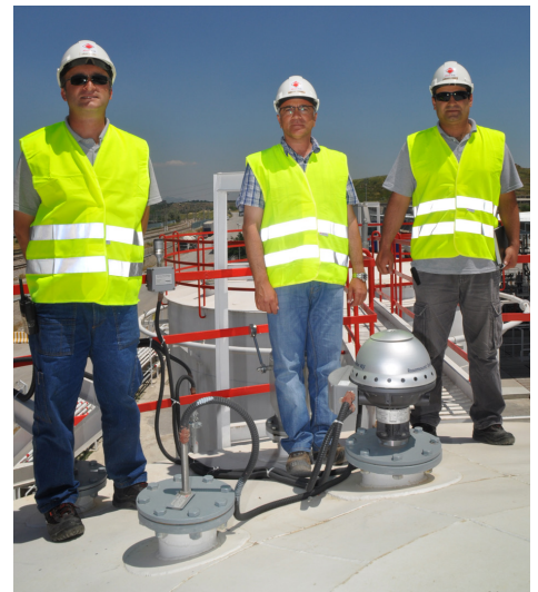
The wireless tank gauging system from Emerson fulfills the high requirements of the Akim Tek team. The system has been up and running since December 2010/January 2011.
