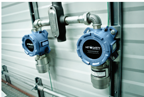
Figure 3. Combustible gas detection sensors.
