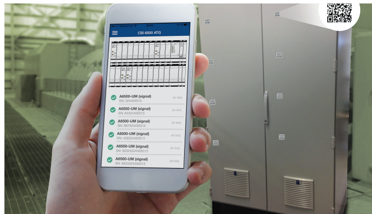
CSI 6500 ATG View delivers asset health information to the user anywhere on the plant network. Scan a quick response code (QR) located on the cabinet and data from the associated rack is viewable on the device screen.
