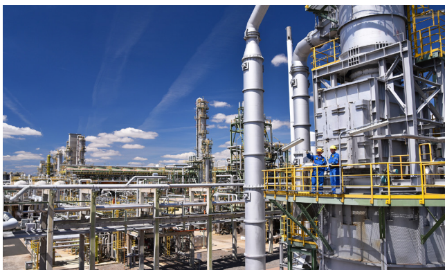
Figure 2. Refineries and general process plants often have many levels, so location systems have to consider height.
