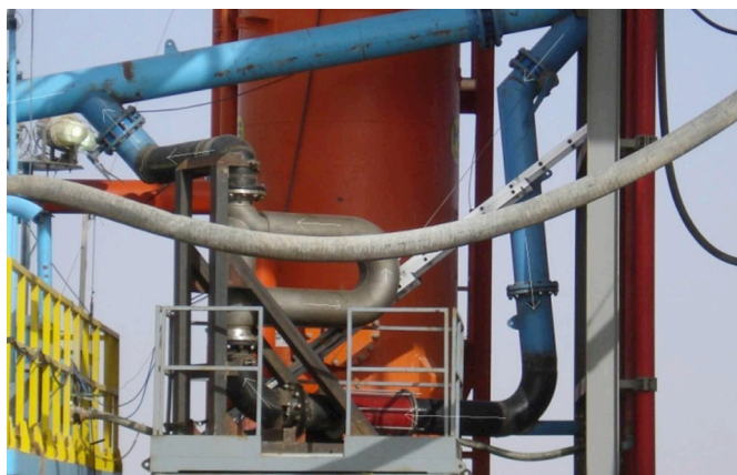
Figure 1. Coriolis meter on a conventional flowline.
