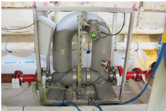
Figure 8. Temporary Coriolis flow meter rigged-up solely for well control purpose offshore Norway.
