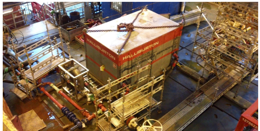
Figure 5. Coriolis flow meter used for automated MPD offshore in Norway.
