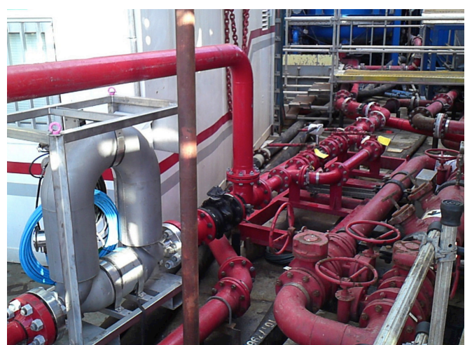
Figure 2. Coriolis installed in an offshore MPD system.
