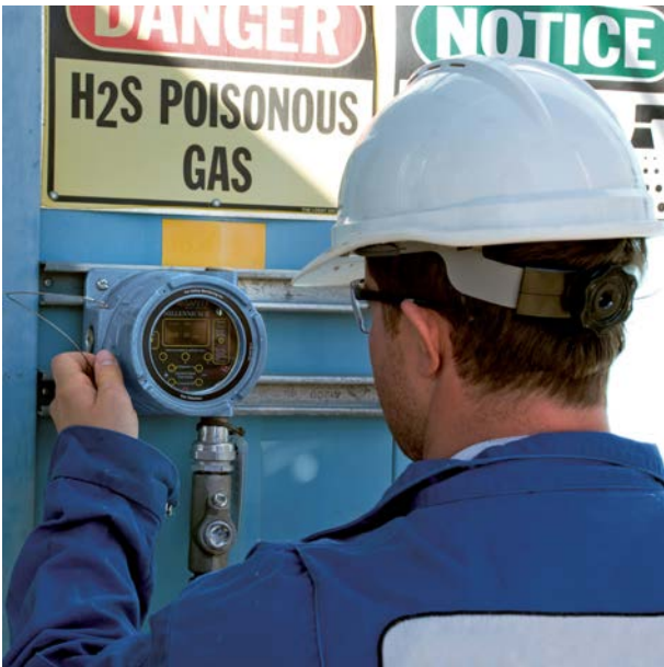
Figure 2. Emerson Rosemount fixed point gas detector.
