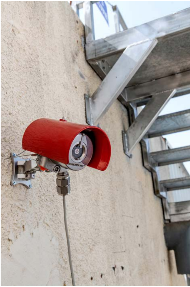
Figure 3. Emerson Rosemount 975 flame detector.
