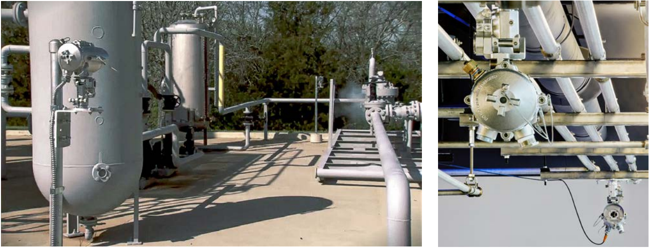
Figure 1. Emerson Rosemount™ open path combustible gas detectors installed.
