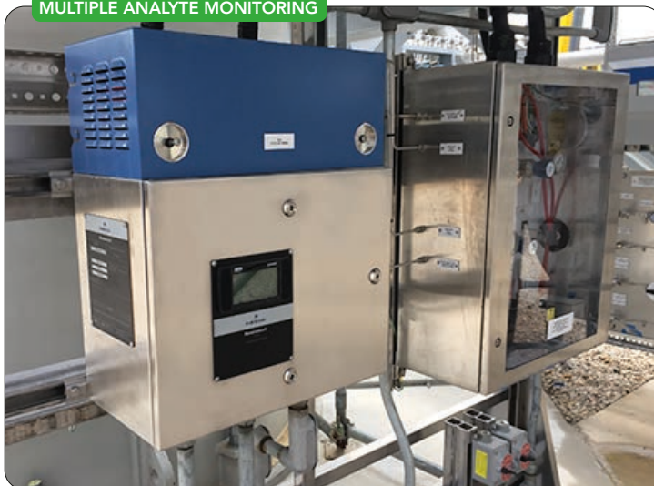
Figure 3. A hybrid QCL/TDL analyzer, such as Emerson's Rosemount CT5100 Continuous Gas Analyzer, can contain up to six laser modules, some of which can measure two analytes.
