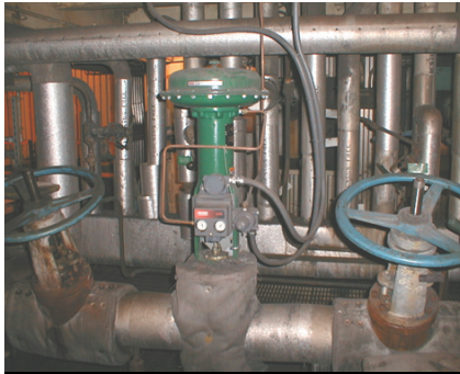
Photo 4. Digital valve controllers eliminated persistent problems with the desuperheating spraywater valves on all four boilers.
