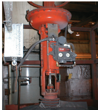
Photo 2. DVC mounted on Unit #1 steam bypass valve on a 10 X 20-inch steam line.
