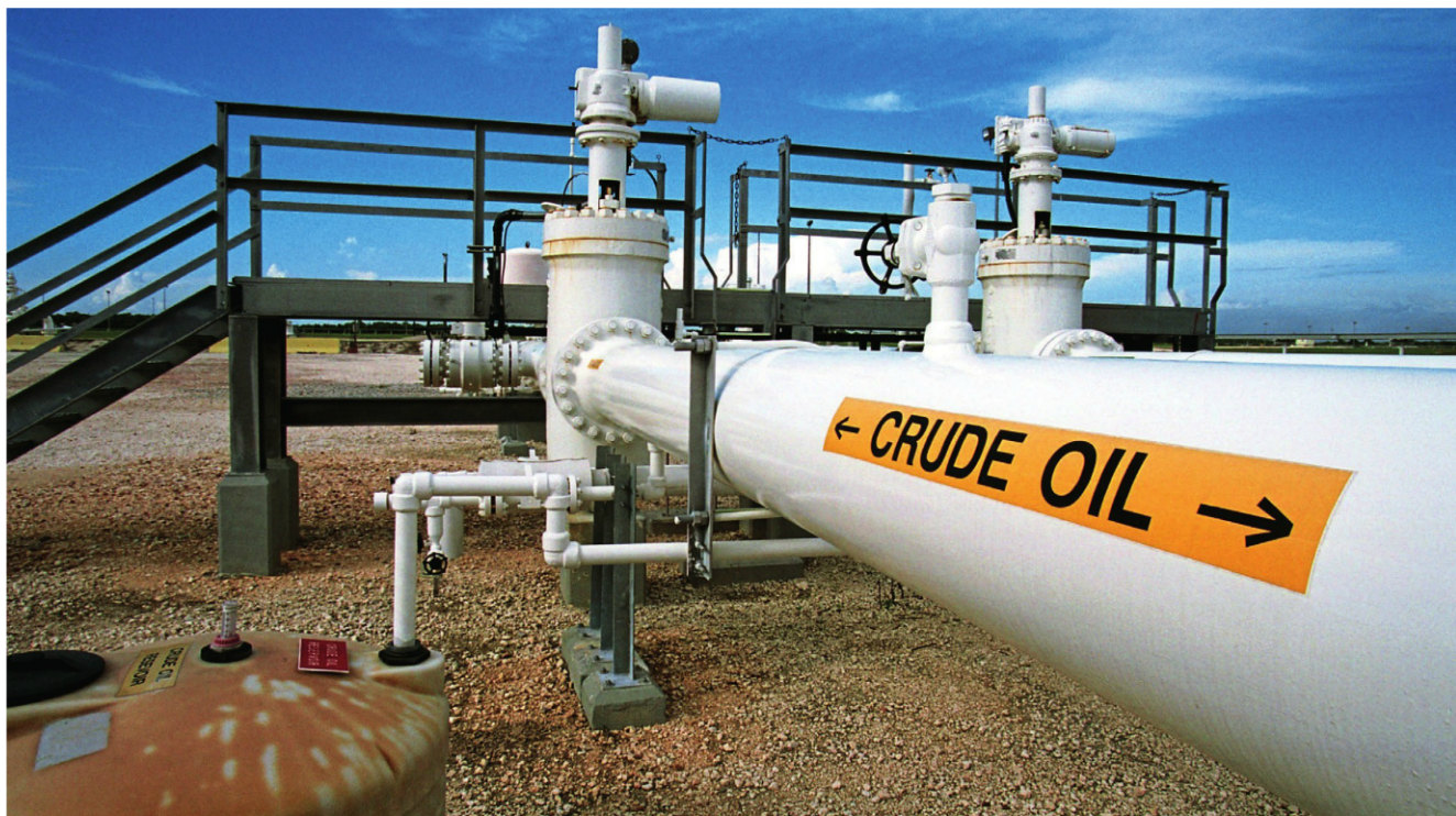
Emerson has significant involvement in the major pipeline network connecting the refineries and terminals of Abu Dhabi, and the pipeline backbone of Malaysia's gas
