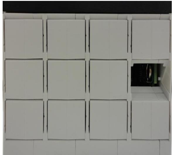
Controller Battery Area
