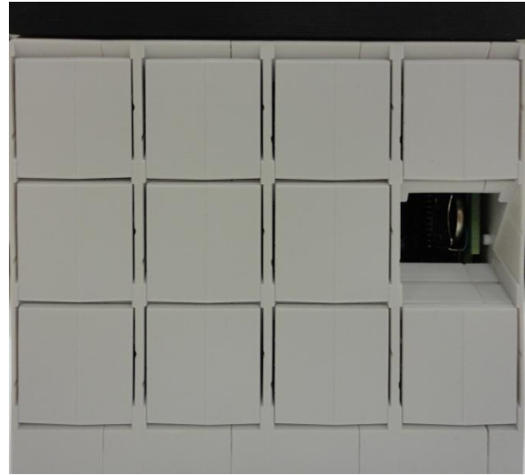
Controller Battery Area
