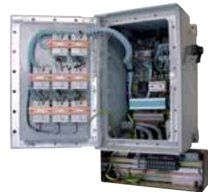
Ex d Panelboard with 8 Branch Circuit Breakers Coupled with Ex e Polyester Junction Box
