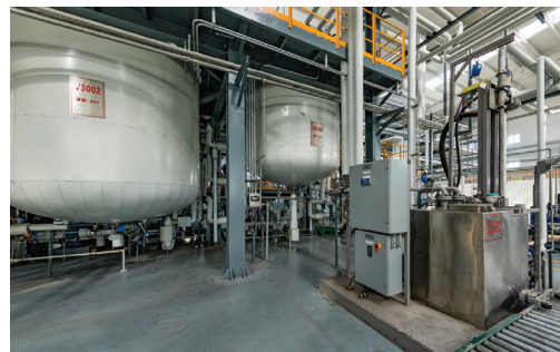
Emerson's Batch Blending Vessels installed at a Lubricant Blending plant in China.
