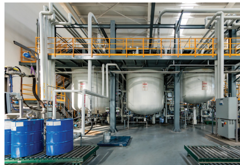
Two 10 ton batch blending vessels and one 5 ton vessel used to blend small volume lubricant batches.
