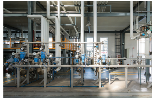
A 4-Loop Simultaneous Metered Blender with piggable discharge header installed in China. Photo courtesy of Copton.
