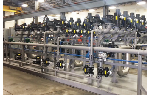
Turnkey Simultaneous Metered Blender undergoing Factory Acceptance Testing.
