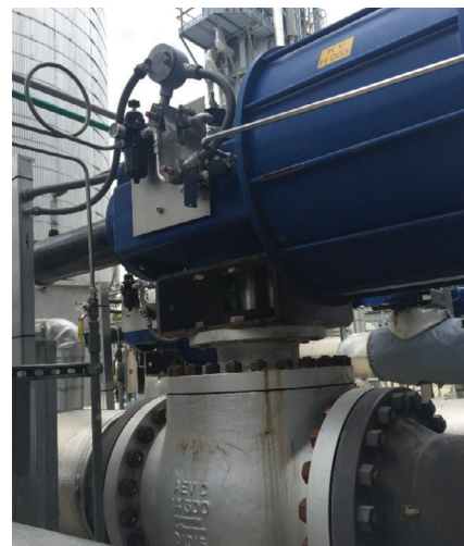
FIGURE 2 Typical switching valve installation in Texas, USA
