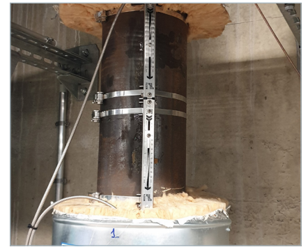
Measuring point with the clamp-on ultrasonic transducers mounted in the Variofix L transducer attachment device on the DN200 hot water pipe.
