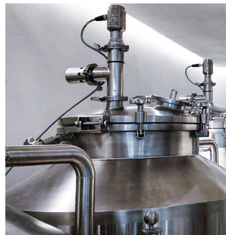
Image 2. The Rosemount 1408H Level Transmitter was connected to a logic control unit (PLC).
