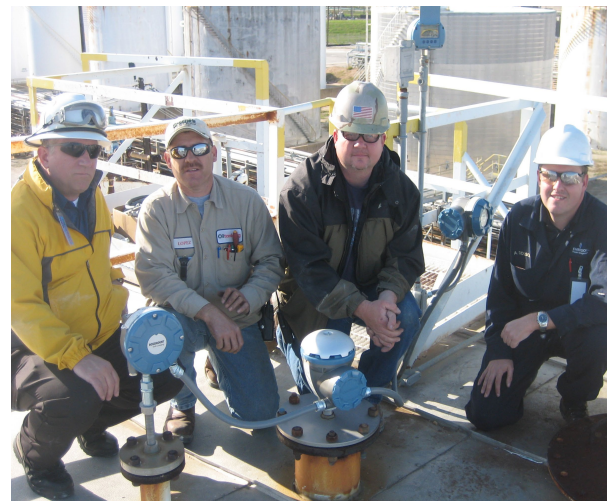
Rosemount Tank Gauging System installed on tank TK3740
