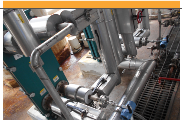
Rosemount 2051 Wireless Pressure Transmitters and 648 Wireless Temperature Transmitters were deployed at the inlet/outlet shell of the heat exchangers to gather data and manage fouling.
