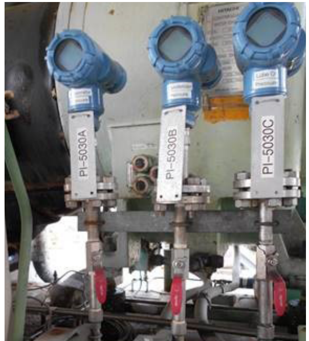
Rosemount 648 Wireless Temperature Transmitters were installed to monitor the efficiency of the chiller system.
