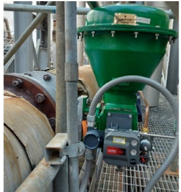
The 12-inch Fisher V150 Vee-Ball Valve with noise attenuator and FIELDVUE DVC6200 installed on-site
