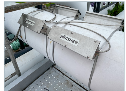
Measuring point with the ultrasonic transducers mounted in Permalok rails on the outside of a DN300 crude oil pipe. Two measuring channels with two pairs of ultrasonic transducers allow for effective compensation of the effects of disturbed flow profiles.
