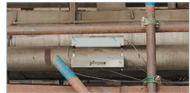
Measuring point with the clamp-on ultrasonic transducers, installed in Variofix C mounting rails.
