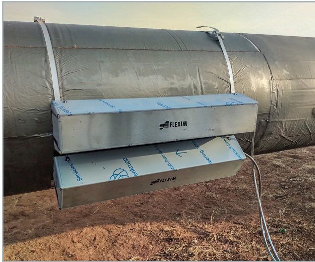
Measuring point with transmitter FLUXUS® F721 and transducers mounted in Variofix C, both in stainless steel.
