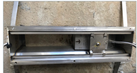
Meter installation with no interruption of flow and no downtime on this 48-inch concrete force main, flowing raw sewage. Straps went around the pipe securely, holding the PermaLok tracks and the transducers tightly with a maintenance-free coupling pad.
