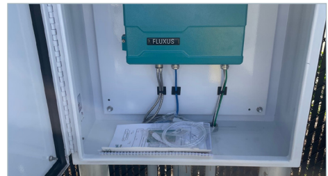
The finished measuring point with its single pair of CDK transducers was up and running in a few hours with no service interruption and no spilling of raw sewage.
