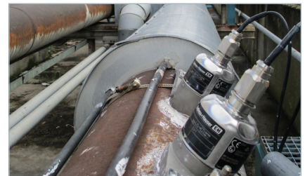
The high-maintenance previous measuring device
