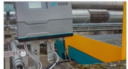
The new flow measuring point with the stationary FLUXUS® F721 measuring transmitter in the foreground and the ultrasonic transducers mounted in the Variofix C in the background
