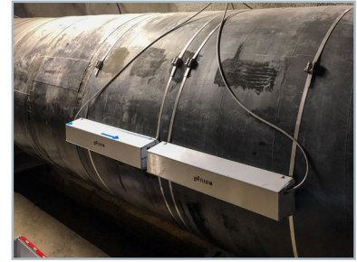
The finished installation with the clamp-on ultrasonic transducers attached to the Variofix C mounting rails (the corresponding counterparts on the other side of the pipe are not visible in the picture).
