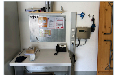
Now a FLUXUS® G722 is used. The synchronous two-channel measurement of the FLUXUS® G722 effectively compensates for the flow profile disturbance. Instead of being installed directly next to the transducers, the transmitter was now installed in a technical room in the tunnel.
