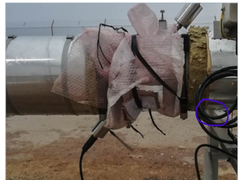
The non-working clamp-on ultrasonic flow measurement system which was intended to measure the reinjected gas quantities at the well.
