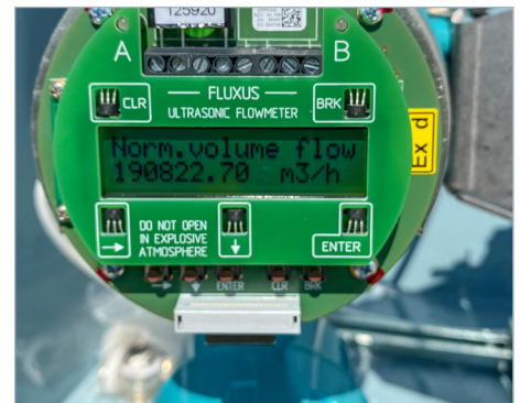
The FLUXUS® G809 is used as a measuring transmitter, here in operation during commissioning.
