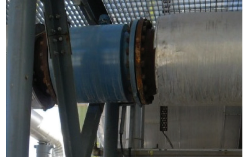
Installed magnetic flow meter in a main brine line.
