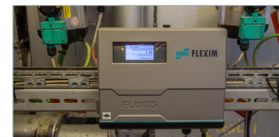
Stationary, clamp-on FLUXUS® F721 ultrasonic flowmeters are used as measuring transmitters.
