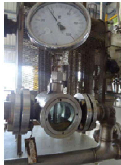
This sight glass and gauge needed to be read and manually recorded at the correct times.
