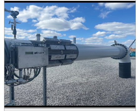
Quad beam measuring point on one of the supplying pipelines
