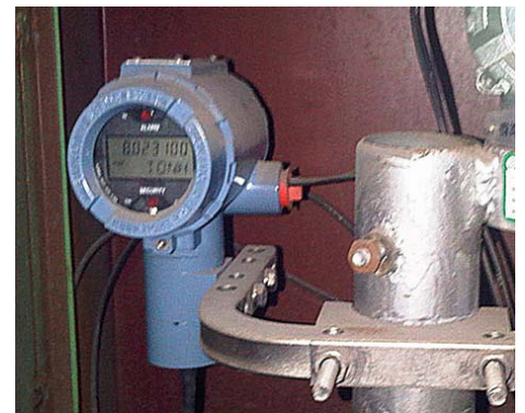
Image 1. Installed Rosemount 8600 Vortex Transmitter
