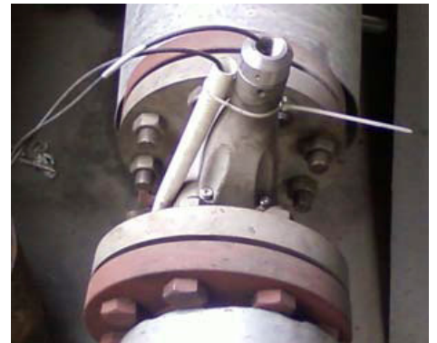
Image 2. Installed Rosemount 8600 Vortex Flow meter
