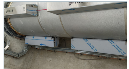
Measuring point with ultrasonic transducers installed in a Variotfix C transducer mounting device on the outside of a DN600 crude oil pipeline. Two measuring channels with two pairs of sensors allow effective compensation of the distorted flow profile.
