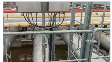
The FLUXUS® H721 is used as the measuring transmitter. The stationary ultrasonic system was specially developed for the non-intrusive measurement of hydrocarbons and, in addition to the volume flow, also measures the density and thus the mass flow.
