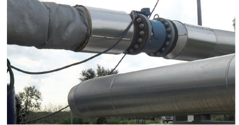
Rosemount 8705 Magnetic Flow Meter installed in the brine line.
