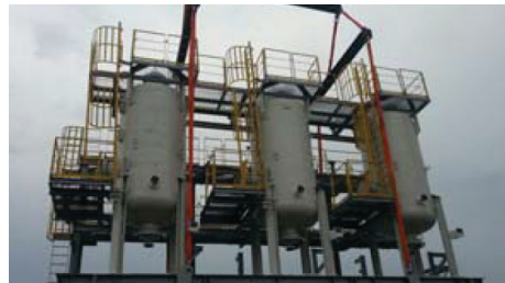
Water demineralization unit mounted in the FLNG plant
