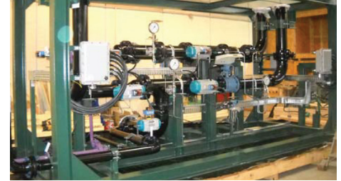
Water Treatment Skid
