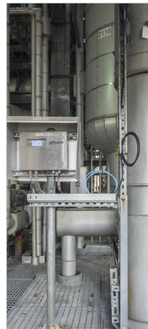
The stationary FLUXUS® F721 ultrasonic systems are used as the measuring transmitters.
