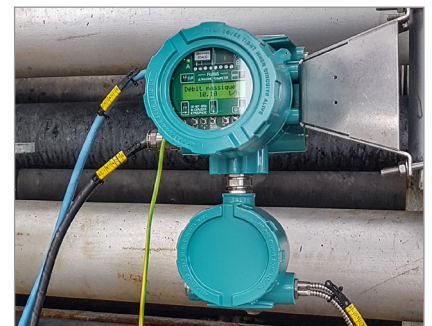
A dual-channel FLUXUS® G809 is used for simultaneous flow measurement on two pipes. Both transducers and transmitters are installed in hazardous area classified ATEX zone 1.
