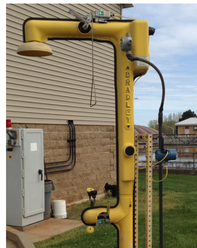
A 702 Wireless Discrete transmitter with TopWorx GO Switches communicate to a Smart Wireless gateway 1000 feet away to alert operators when the shower or eyewash station is activated.
