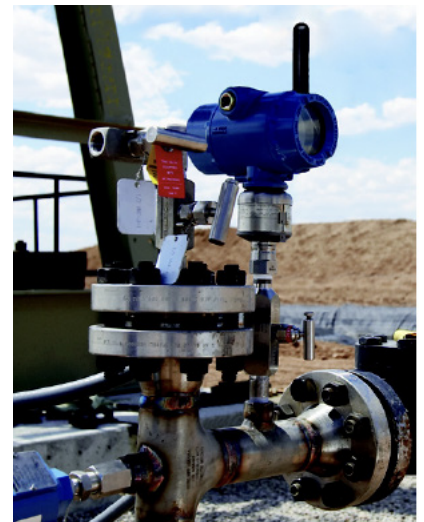
The Rosemount™ 3051S Wireless Pressure Transmitter Installed
