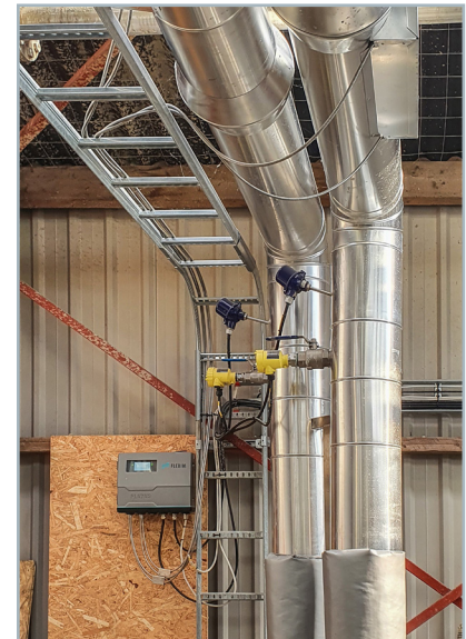
Measuring point with a stationary FLUXUS® F721 measuring transmitter and the transducers (integrated into the insulation)
