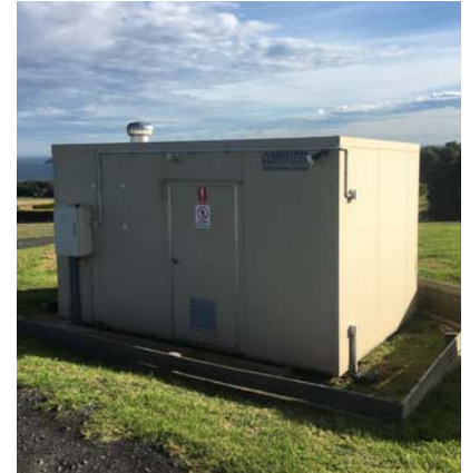
Chloramination monitoring at remote site
