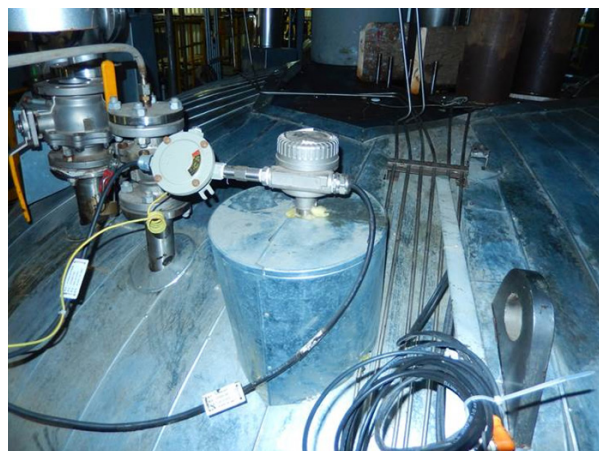
Rosemount 2130 SIL2 Vibrating Fork Level Switch mounted on top of the reactor
