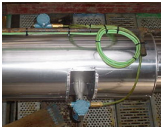
A Rosemount 8800 Dual Vortex installed.
