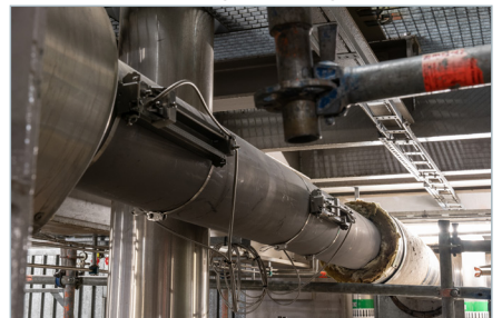
Measuring point with clamp-on transducers mounted on the outside of the pipe.
