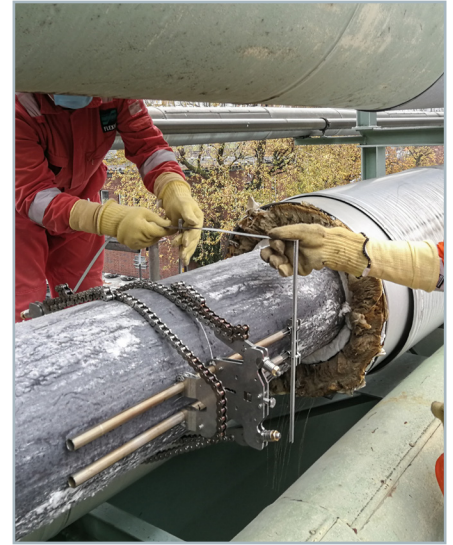
Installation of the high-temperature Wave-Injector® transducer mounting devices on a hot pipe. The insulation only needs to be removed temporarily from the pipe to install the ultrasonic transducers.
