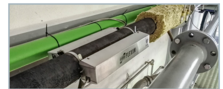
The insulation only needs to be temporarily removed to install the clamp-on ultrasonic transducers on the pipe.
