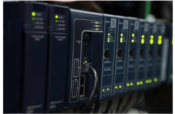
PACSystems RX3i controllers in redundant configuration interface with field instrumentation.
