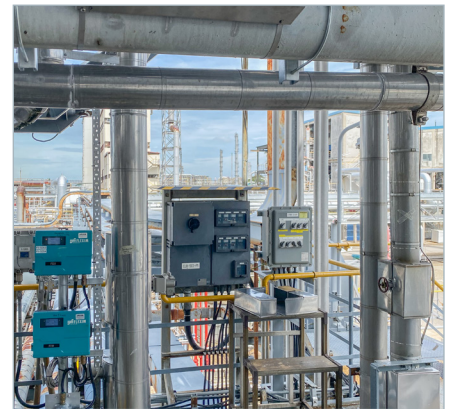
Measuring point with the clamp-on ultrasonic transducers, installed in a Variofix C mounting rail. In the background two FLUXUS® F721 transmitters.
