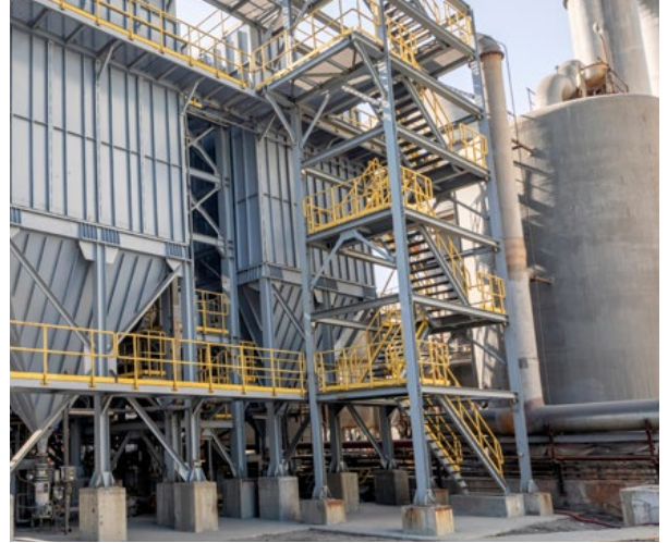
Dust collector air bag filter.
